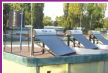
SOLAR WATER HEATER
