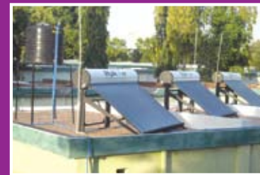
SOLAR WATER HEATER
